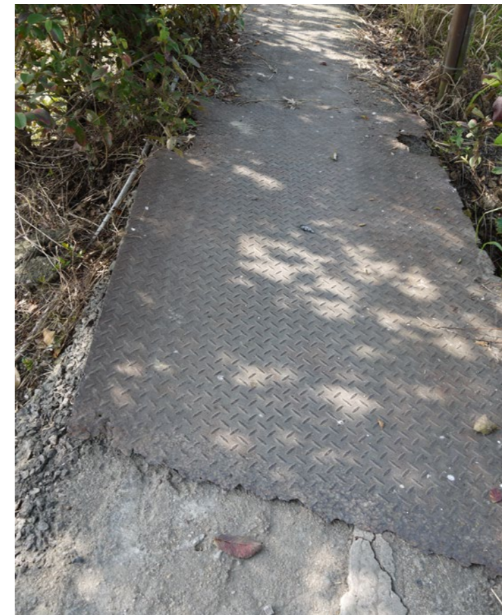
Potential hazard area
